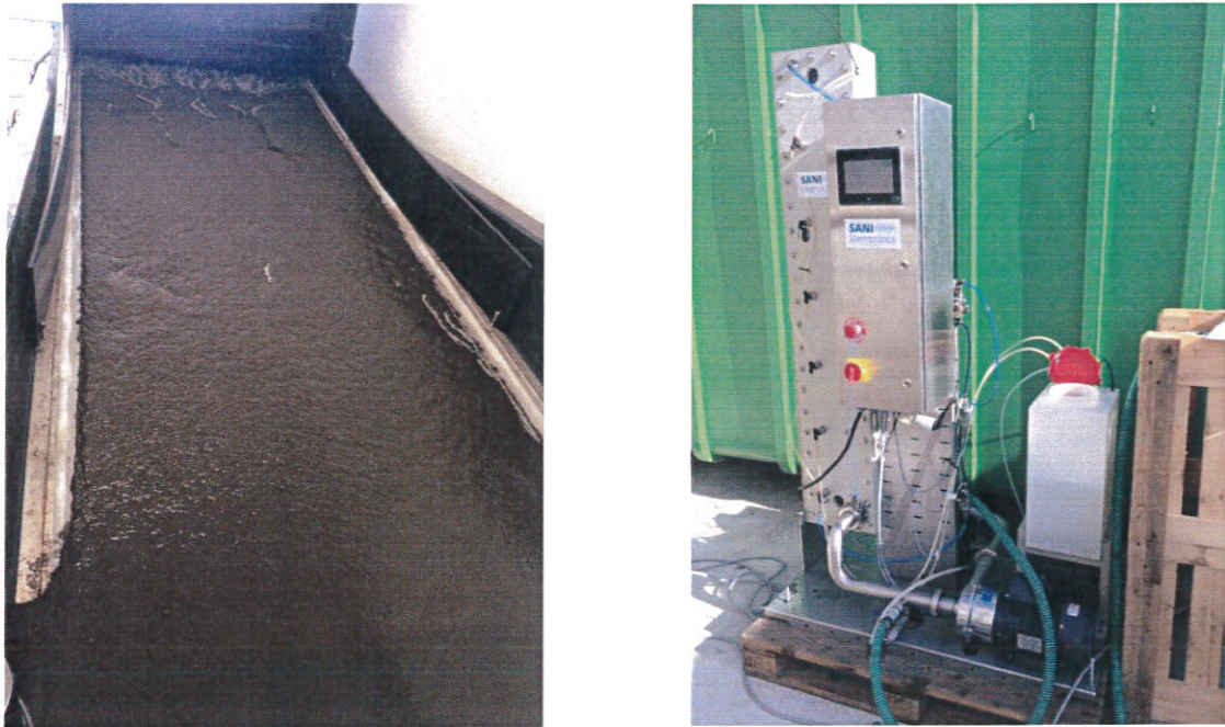
Figure 3. Left photo show filter A: belt filter. Right photo shows filter B: cross-flow membrane filter.
